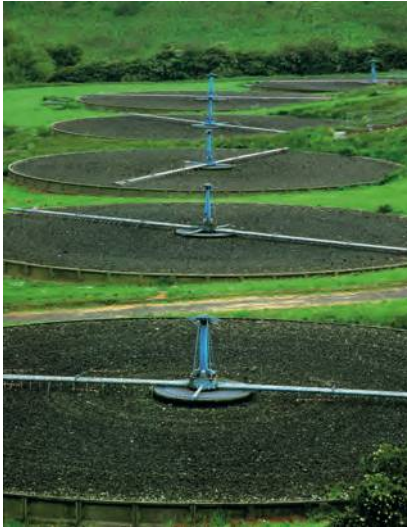
This is a trickling filter system at a sewage plant in Yorkshire, England. Have you visited the waste treatment plant in your community?
